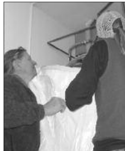
Adele Bachman and Brooke Murphy learn how to wrap a water heater at the Mt. Crested Butte workshop.
